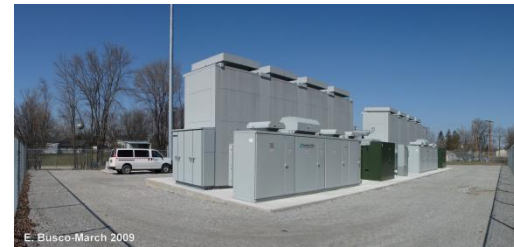
Sodium Sulfur Battery 2 MW
